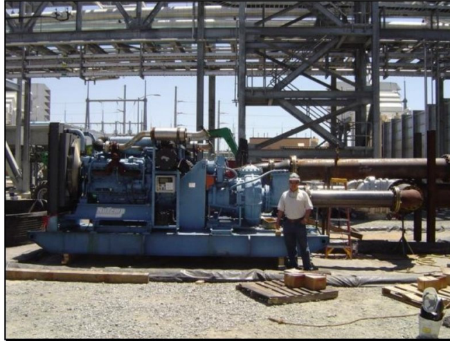
Chemical Cleaning System – 5,000 gpm
