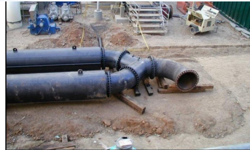
LOK Energy Temp Exhaust Pipe
